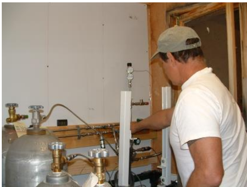
Conditioning and filling cylinders.
