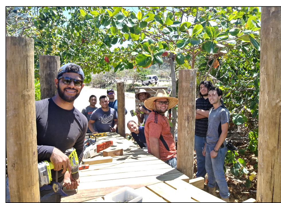
Figure 7. UPR students working on the construction of a wooden boardwalk in the Isabela sand dune system.
