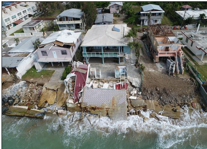
Figure 3. Massive structural damage in Puerto Rico as a result of waves and storm surge from Hurricane María in 2017.
